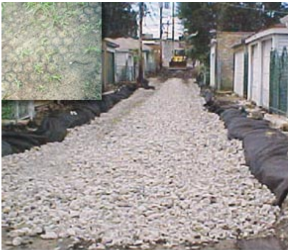
The alley, constructed of a rigid grid system and gravel, allows rainwater to soak into the ground. Close up of finished system upper left corner.
