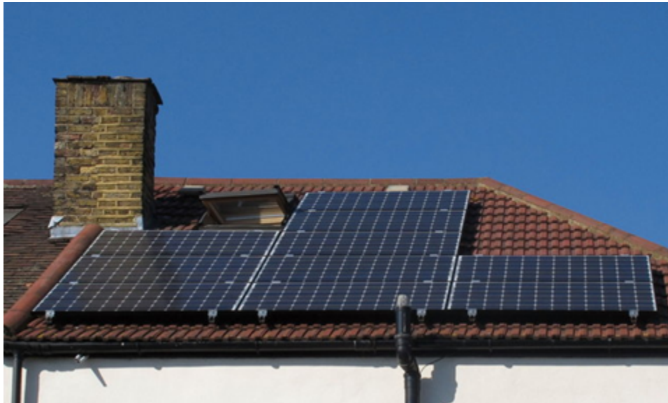
Figure 1: "Installation of solar PV panels - panels in place" by David Hawgood is licensed under CC BY-SA 2.0.
